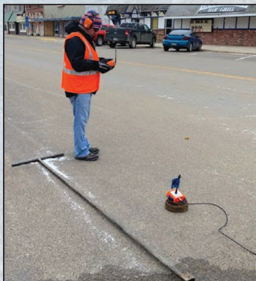
Chuck Mischel of ND Rural Water utilizing leak correlation equipment to pinpoint a utilities water leak.
