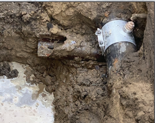
This leak was found on an abandoned lead service line.
