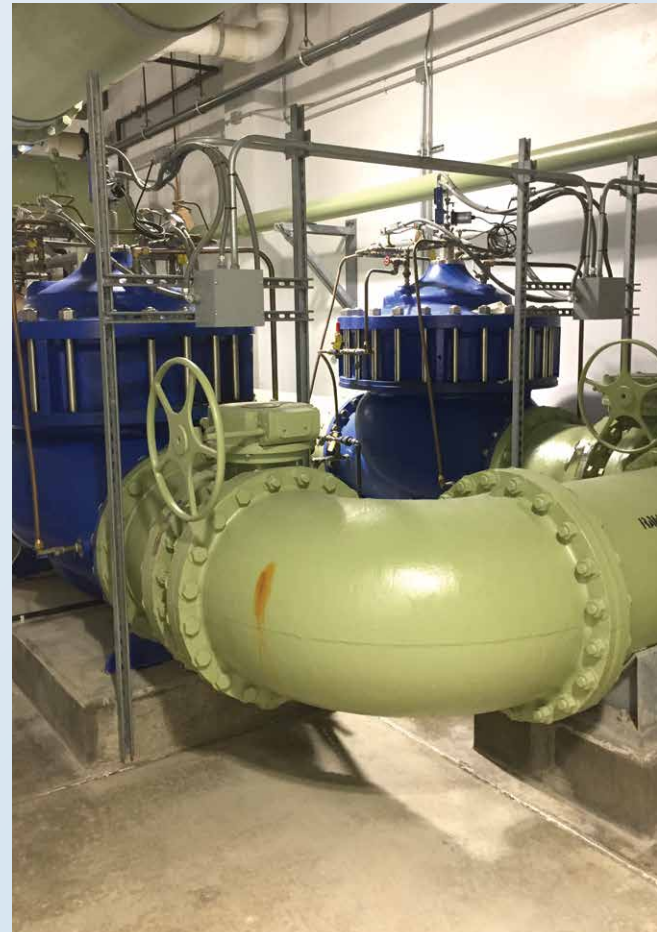
Increased demand requires increased complexity of the distribution system. This valve is located in Southwest Water Authority's Dickinson plant.
